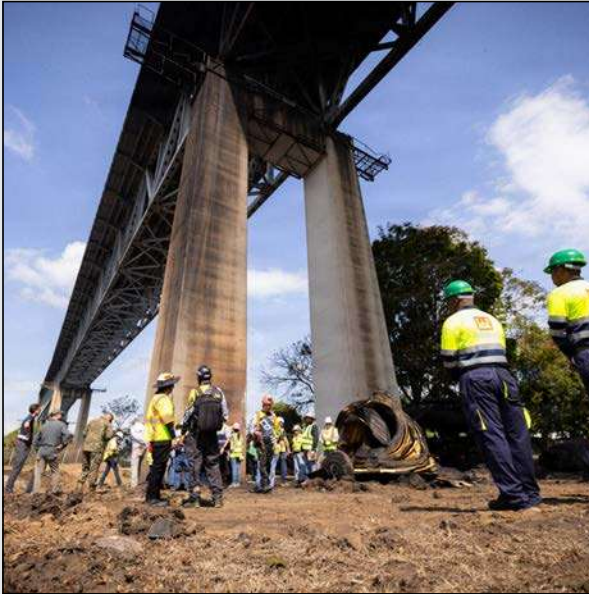
The US Army Corps of Engineers and Panamanian partners conduct an engineering assessment of the Bridge of the Americas in Panama, April 10, 2026 (US Army photo by Rydell Tomas Jr.).
